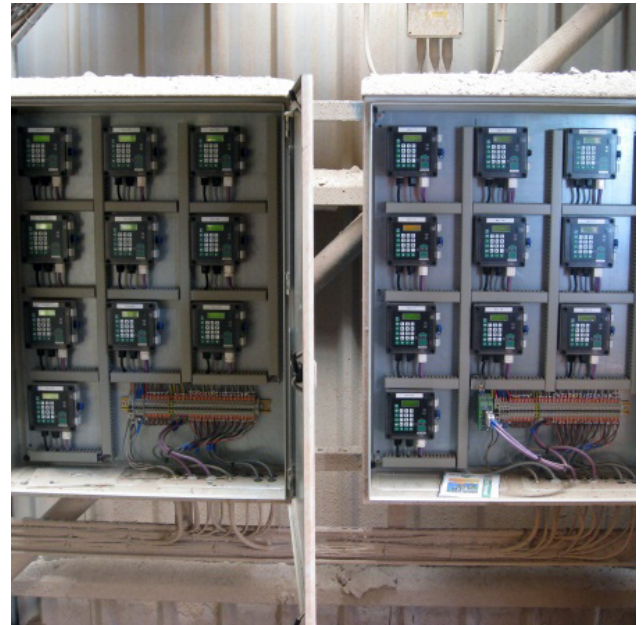
20 Blackbox Units housed in control cabinet.
